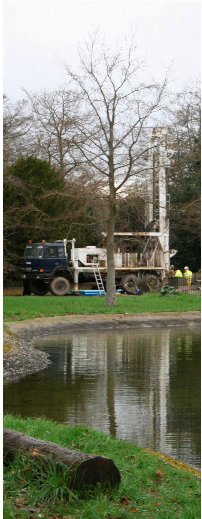
Hydreq Gryphon 16 tonne rig drilling a water supply borehole to supply a lake and irrigate a garden.
