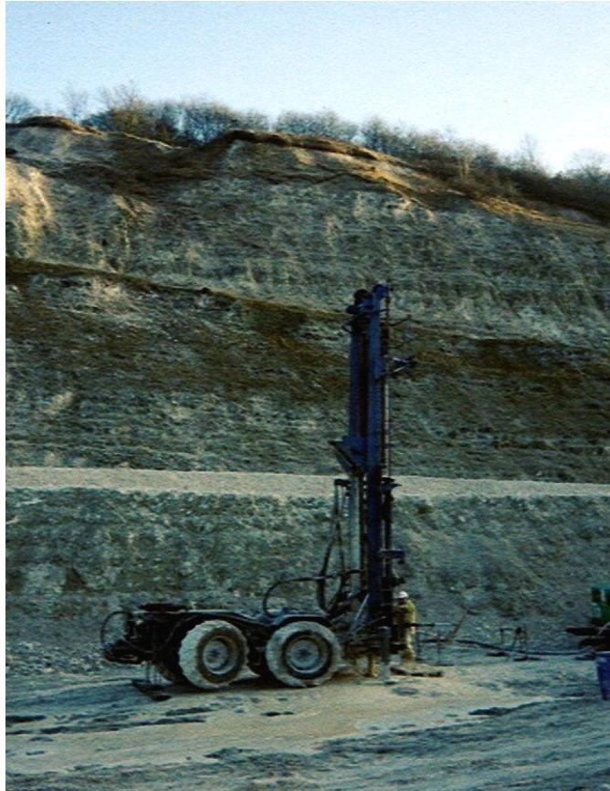
Drilling through Lower Chalk into the Upper Greensands in a former chalk quarry for a domestic water supply in Dorset.
