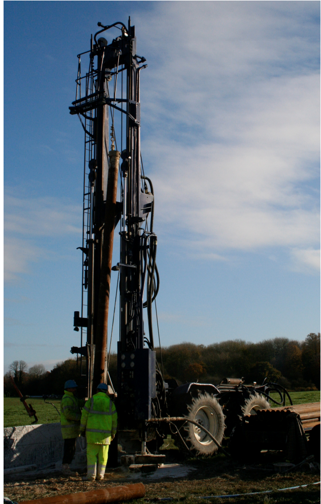
Hydreq Gryphon 10 tonne rig drilling a borehole through Chalk to supply water to a dairy.
