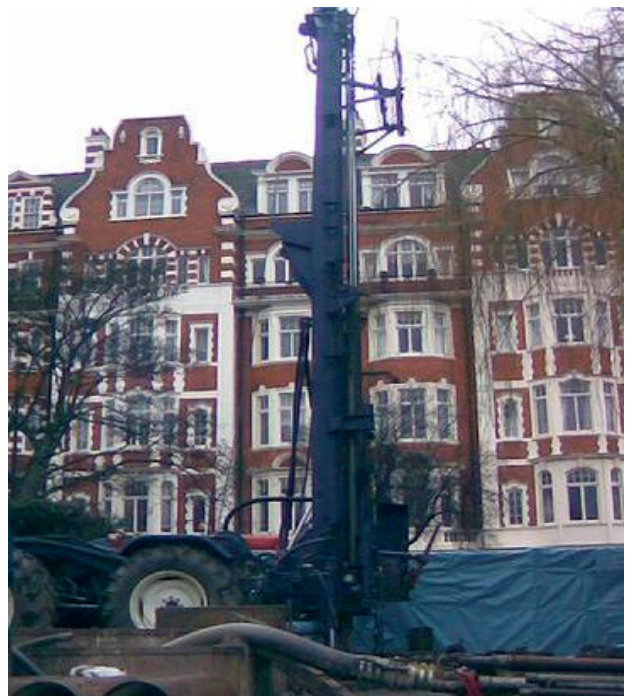
Hydreq Gryphon 10 tonne rig drilling a 140 metres deep water supply borehole in central London
