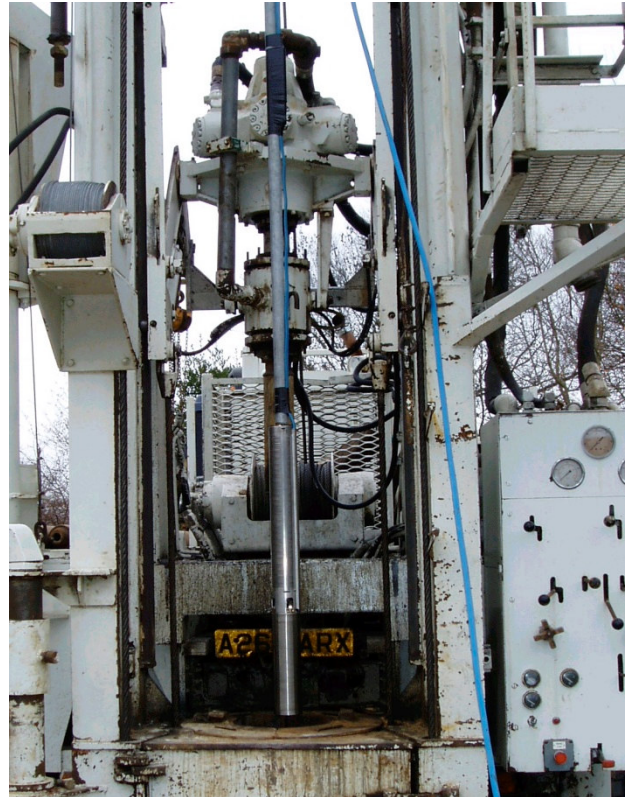
Pump installation for a domestic supply in Surrey.
