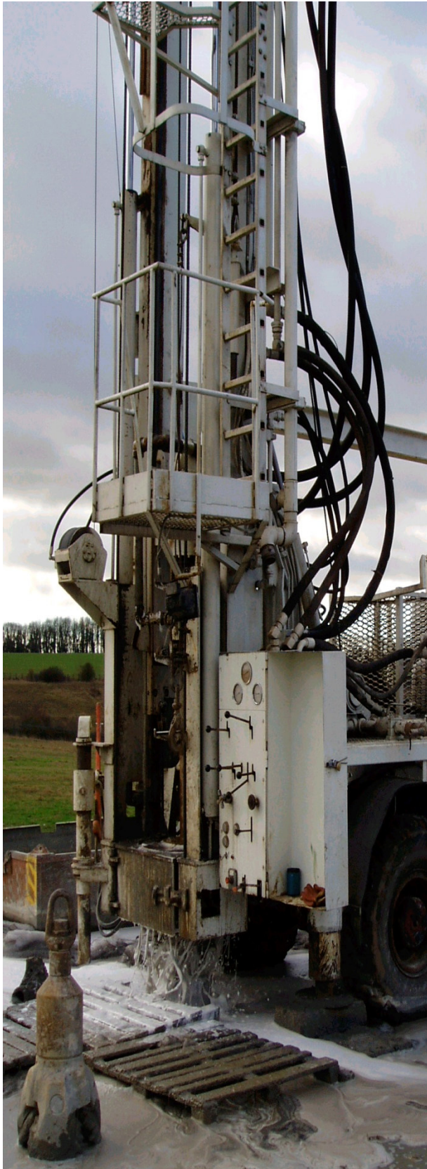
Hydreq Gryphon 16 tonne rotary rig foam drilling through limestone for a bottled water supply borehole.
