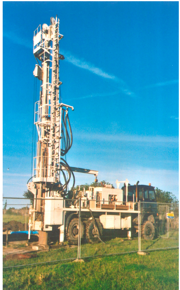
Hydreq Gryphon 16 tonne rotary rig drilling a 140 metres deep limestone borehole in Gloucestershire.
