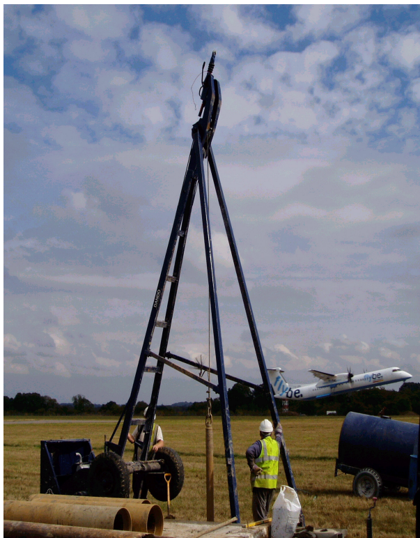
Dando 3000 percussion rig drilling a water sampling borehole for a major international airport.
