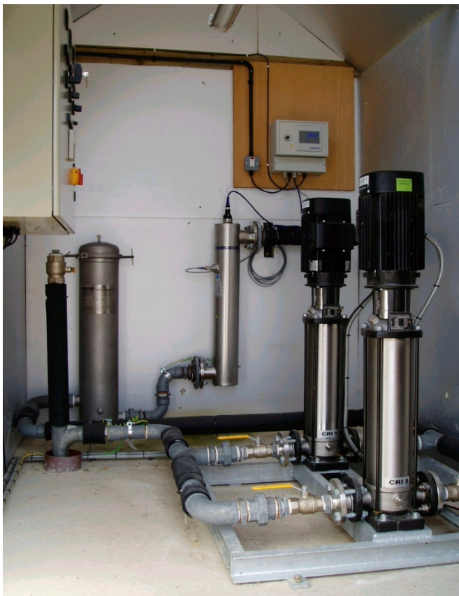
Twin booster pump set with ultraviolet and filter cleansing system for a farm dairy and nearby houses.
